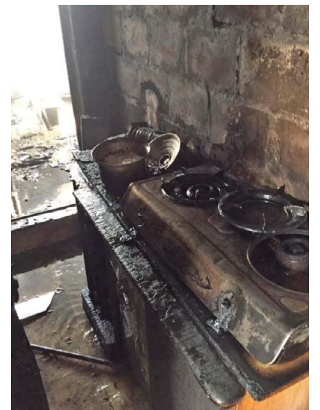
Damage seen inside a Sulaibiya house after a fire was put out.
