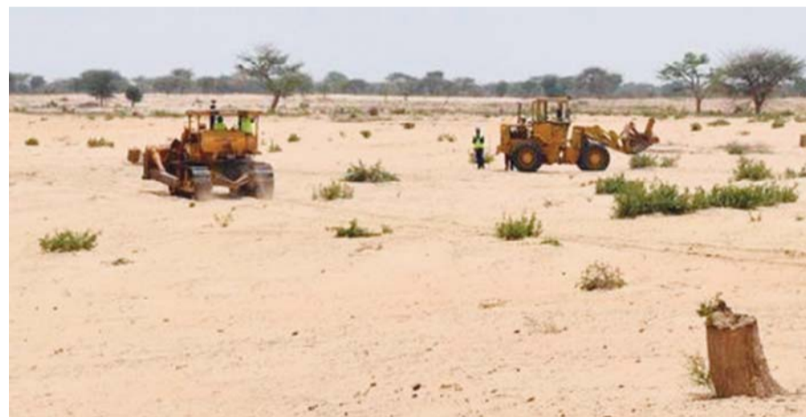
SENEGAL: Bulldozers prepare a field for construction on what is slated to be Senegal's largest solar plant in Santhiou Mekhe on July 11, 2016. —AFP
