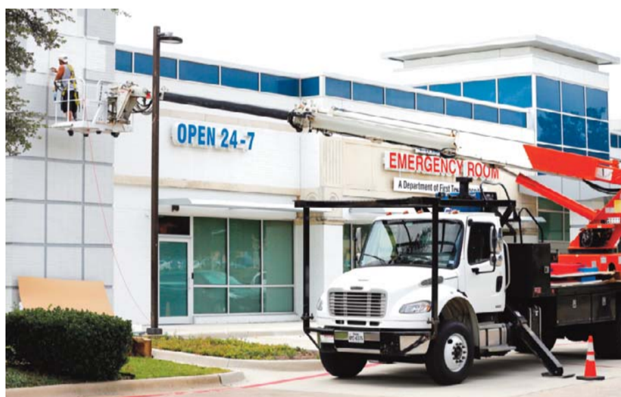
RICHARDSON, TEXAS: A worker makes repairs to an exterior wall of a First Choice Emergency Room on Thursday. —AP
