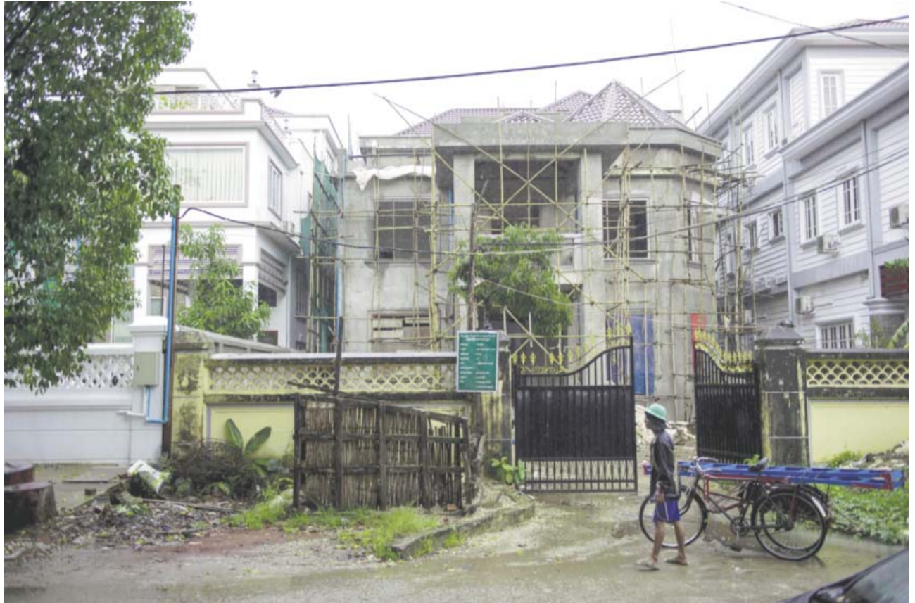
YANGON: A man wheels a bicycle outside a house under-construction in Yangon's residential district yesterday. — AFP
