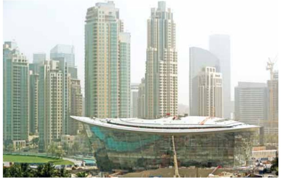
A picture taken June 20, 2016 shows the Dubai Opera House under construction in downtown Dubai.
