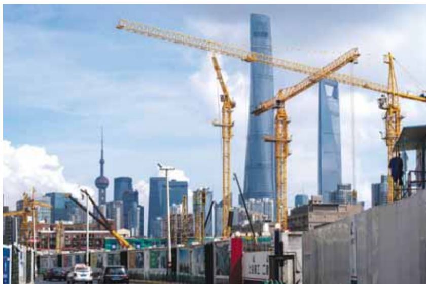
SHANGHAI: Cranes work at a construction site near skyscrapers in the Lujiazui financial district of Shanghai. A Chinese official tried yesterday to reassure companies and investors that China's economic growth is stable despite unexpectedly weak July activity but acknowledged it faces pressure from lackluster global demand. —AP
