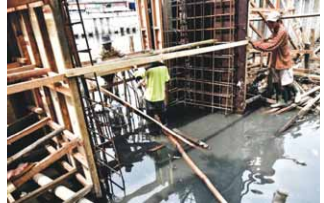
JAKARTA: Laborers work on finishing a riverbank construction project in Jakarta yesterday. Growth in the resource-rich nation has been slipping in recent years due mainly to a slowdown in demand for its key commodity exports - such as coal and precious metals - particularly from Asian powerhouse China. —AFP
