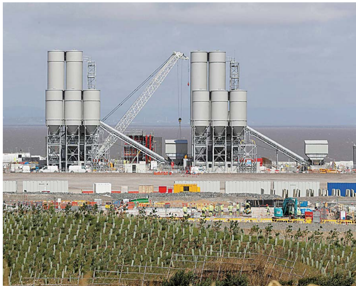
LONDON: The Hinkley Point C nuclear power station site undergoes construction near Bridgwater, England. —AFP
