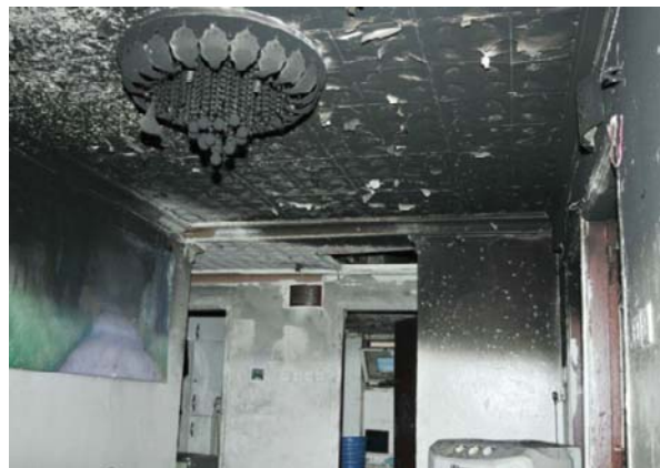
A picture from inside the Jahra apartment taken after the fire was extinguished.
