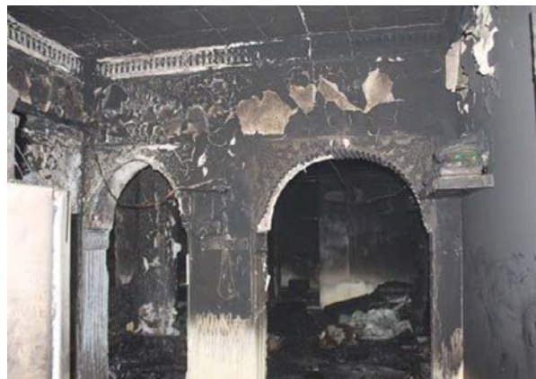
KUWAIT: Damage left by flames inside a house in Sabahiya, where a fire left a woman dead, while her husband and son were hospitalized.
