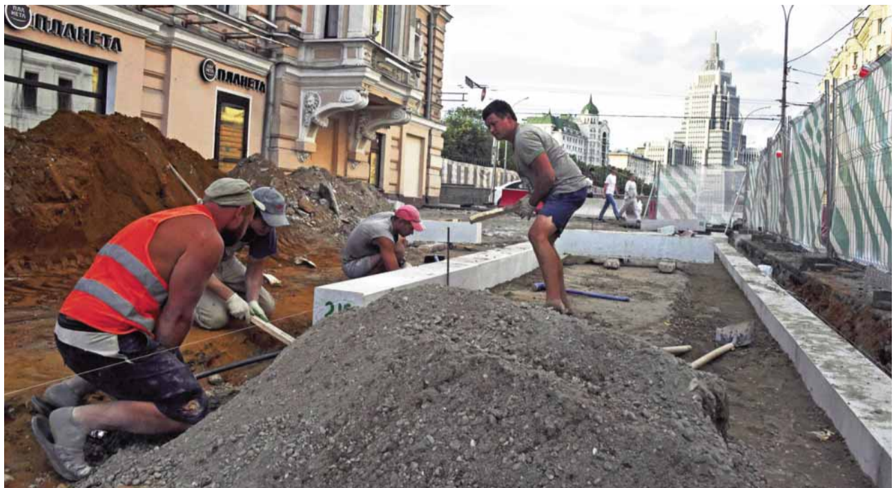
MOSCOW: Municipal workers set up a new pavement in central Moscow on July 10, 2016.
