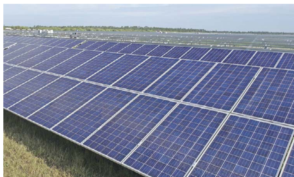
PUNTA GORDA, United States: A solar farm under construction in Punta Gorda, Florida where enough energy will be produced to power 21,000 homes. — AFP photos
