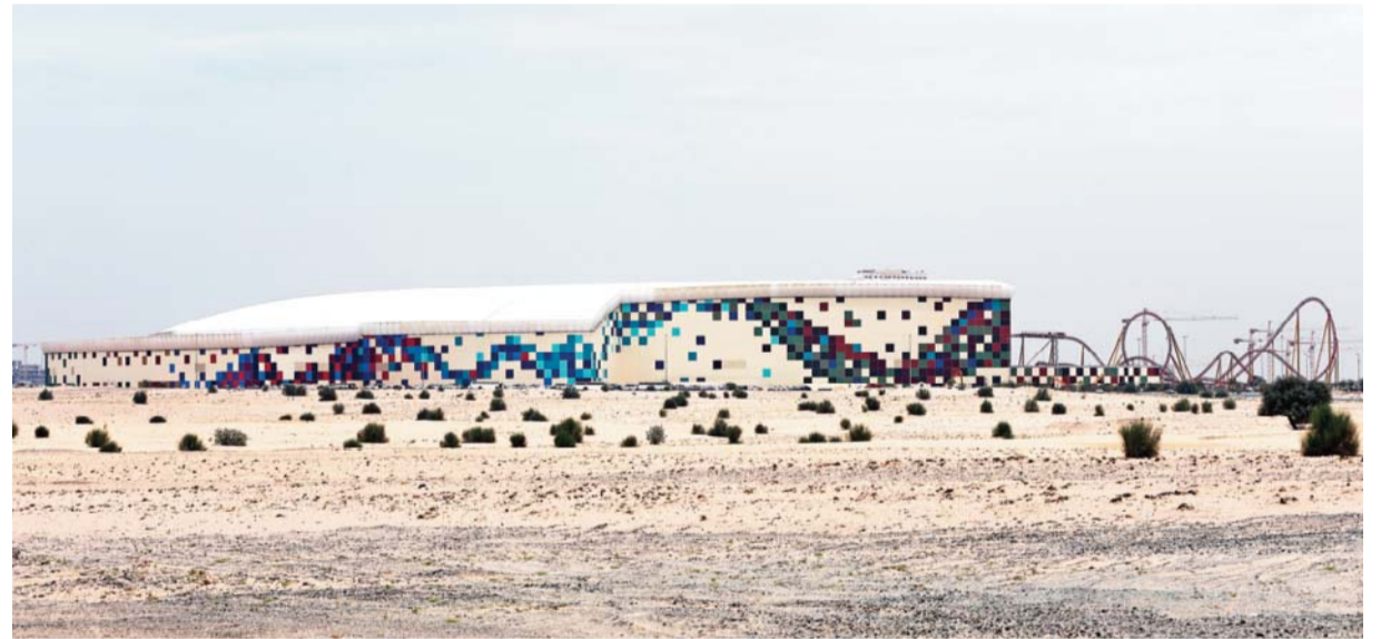
The final steps of construction work are seen at the IMG Worlds of Adventure complex in Dubai.
