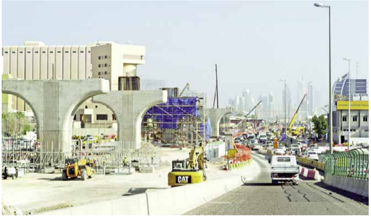
KUWAIT: Photo shows one of Kuwait's gigantic projects being implemented within the state development plan. — KUNA
