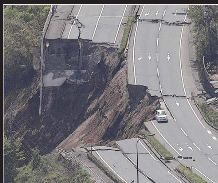
The aerial view shows a collapsed road after an earthquake in Minami-Aso, Kumamoto prefecture yesterday. —AFP
