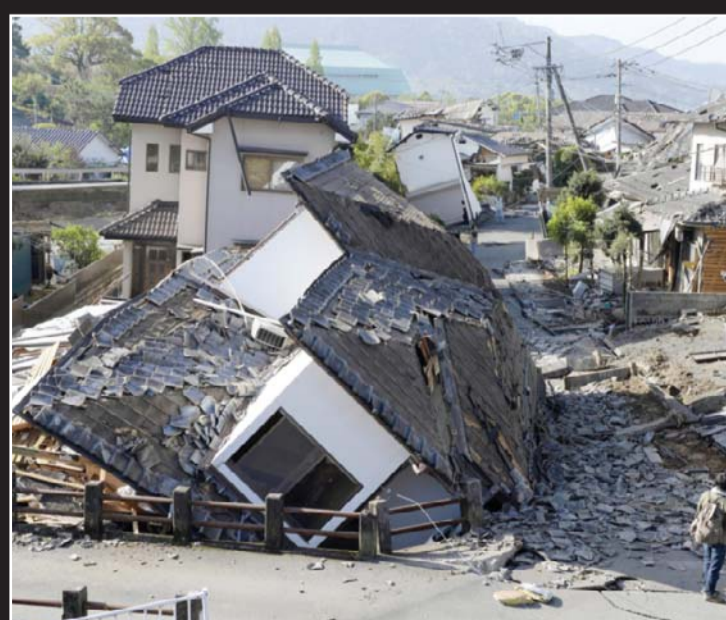
Houses are seen destroyed after an earthquake in Mashiki, Kumamoto prefecture, southern Japan yesterday. — AP
