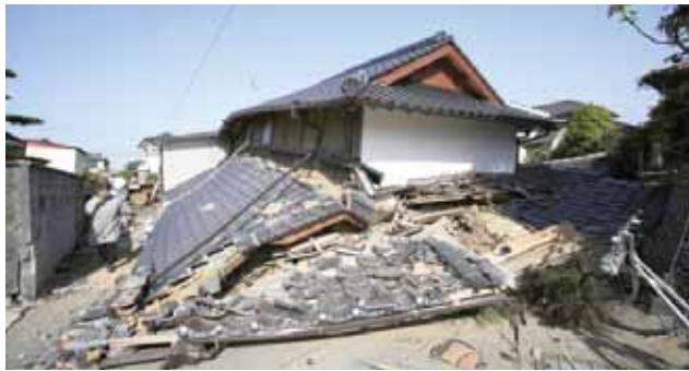
MASHIKI: A resident walks by a collapsed house in Mashiki, Kumamoto prefecture, southern Japan, yesterday. Aftershocks rattled communities in southern Japan as businesses and residents got a fuller look yesterday at the widespread damage from an unusually strong overnight earthquake. — AP
