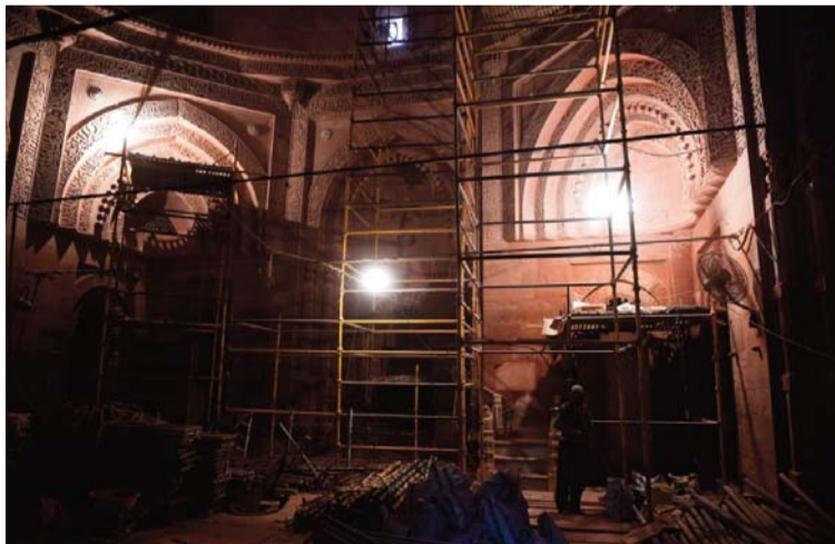
An Indian laborer stands amidst ongoing construction inside the Zamait Khana Mosque at the Dargah of Hazrat Nizamuddin Auliya in the Nizamuddin area.
