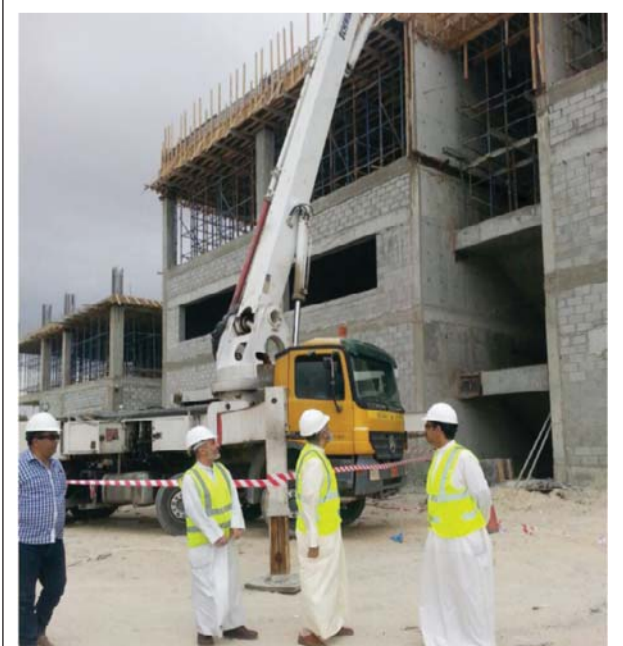
KUWAIT: Deputy director for projects' execution at the Public Authority for Housing Welfare (PAHW) Ali Al-Hubail yesterday toured the Wafra housing project to check on the work progress there.
