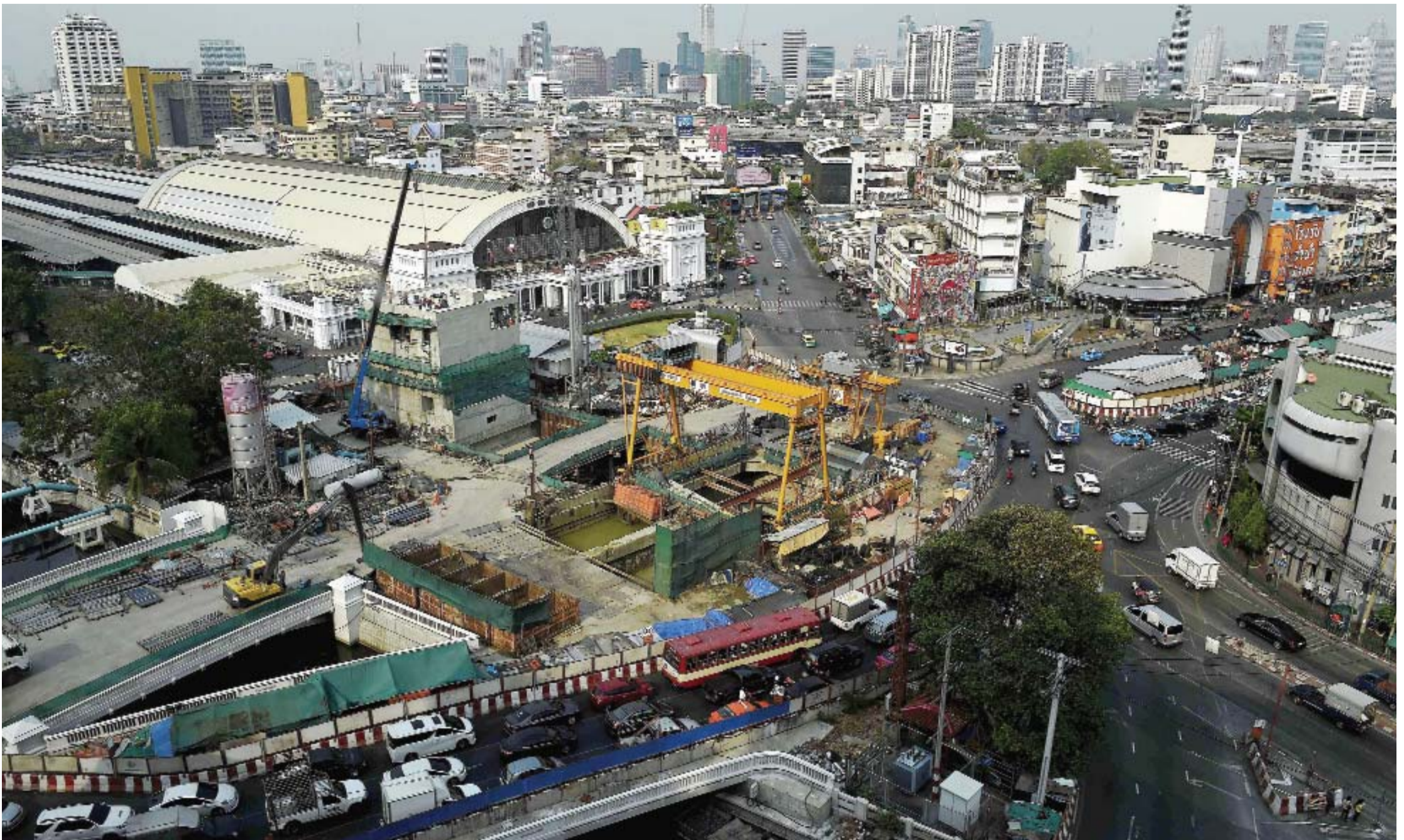
BANGKOK: This picture taken shows a construction site (center) along the current extension of the Metropolitan Rapid Transit (MRT) subway 'Blue Line' into Bangkok's historic district of Chinatown, next to Hua Lamphong's central railway station (left). The Blue Line is the MRT's only line currently in operation, running from the central Hua Lamphong train station to the north of Bangkok and was opened in 2004 as Bangkok's second public transit system. The MRT serves hundreds of thousands of passengers each day, allowing them to escape the city's famously-chaotic traffic, and currently has 18 operational stations along 20 kilometers of underground route. — AFP
