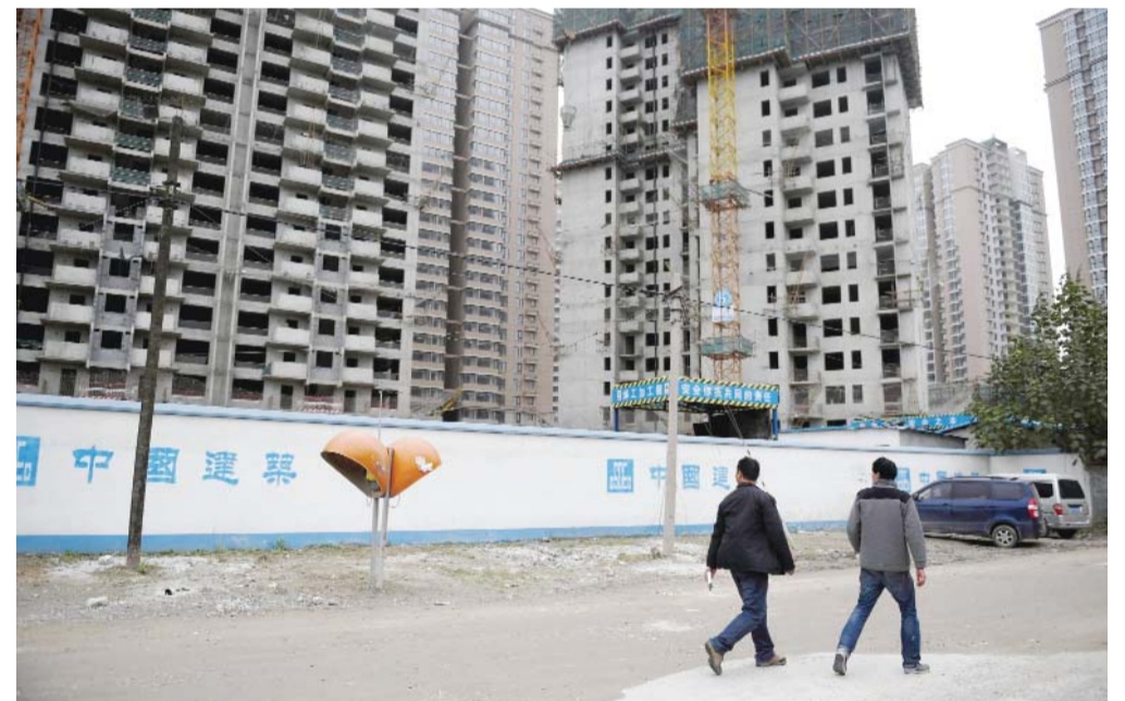
BEIJING: Two men walk past a construction site for apartment buildings in Beijing yesterday. China's leaders will gather today to hash out a new Five Year Plan to battle slowing growth, and analysts say they must choose between chasing a traditional GDP target and embracing reforms such as to the "one child policy" to help the country develop its full potential. — AFP
