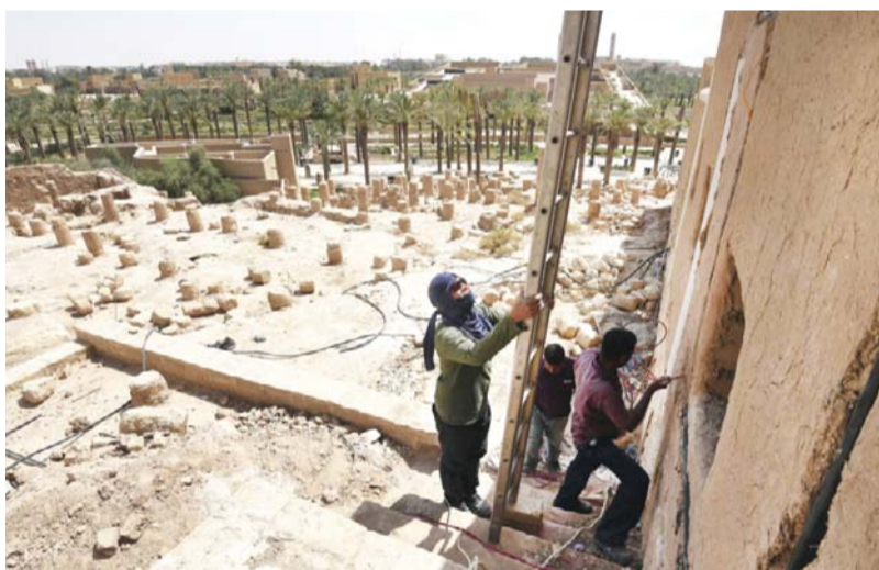
Asian laborers restore an old building in the historical UNESCO World Heritage Atturaf district.
