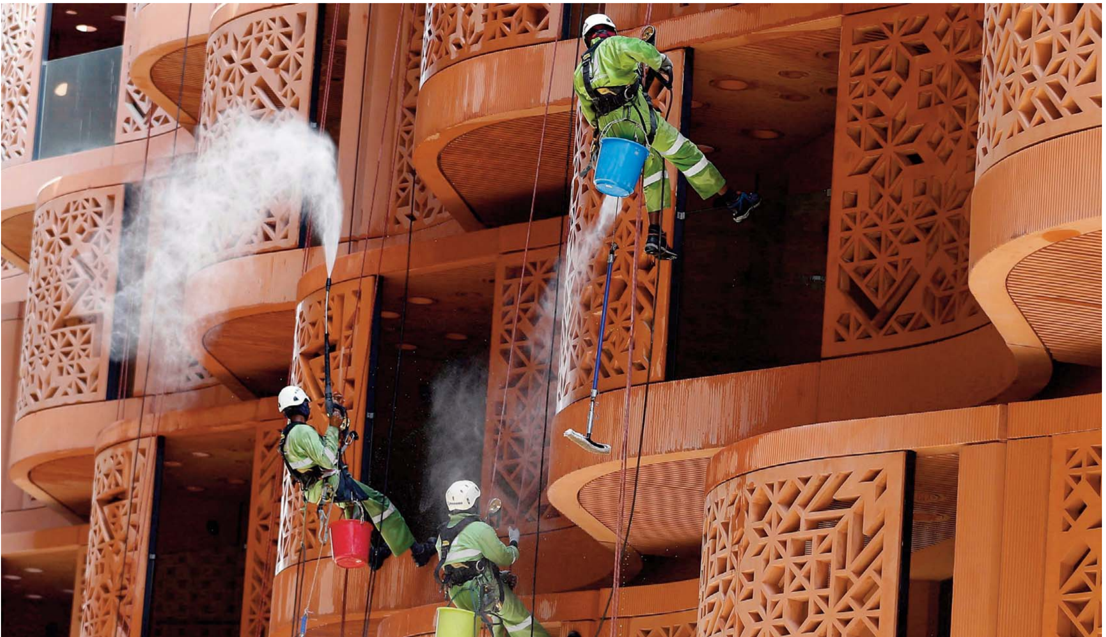
Workers clean buildings in Masdar City on the outskirts of the emirate of Abu Dhabi yesterday. Masdar City is a high-density, pedestrian-friendly development where current and future renewable energy and clean technologies are showcased, marketed, researched, developed, tested and implemented. — AFP
