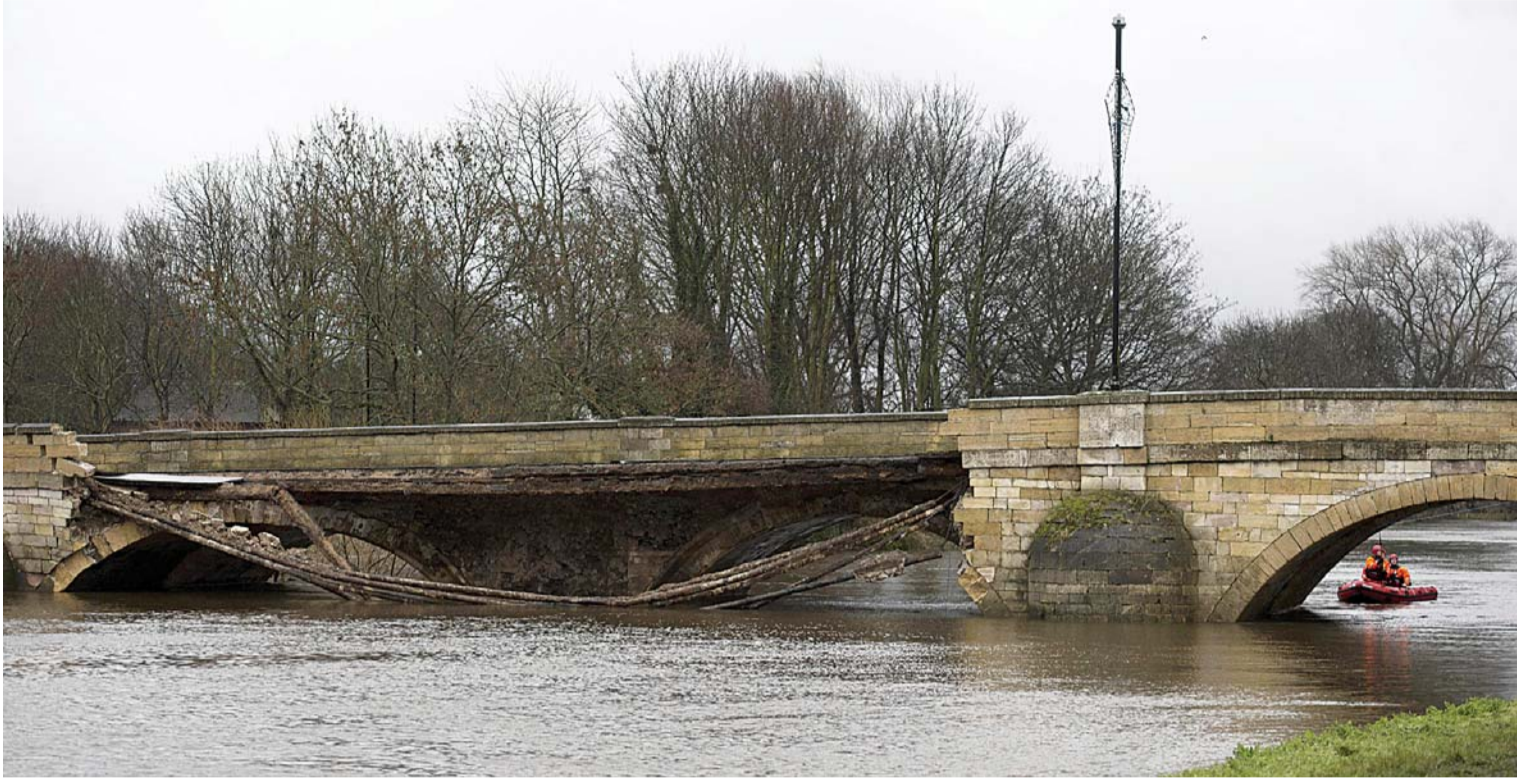
TADCASTER: Members of the emergency services assess the damage to a bridge caused by floodwater over the River Wharfe. —AFP
