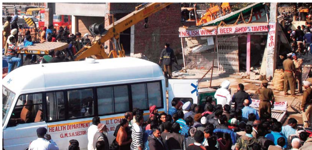
CHANDIGARH: Indian rescuers search for victims in the rubble of a collapsed building. — AFP
