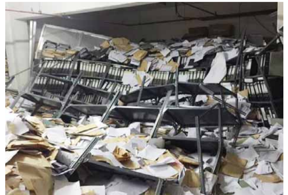
Damage seen at the site where the collapse was reported.
