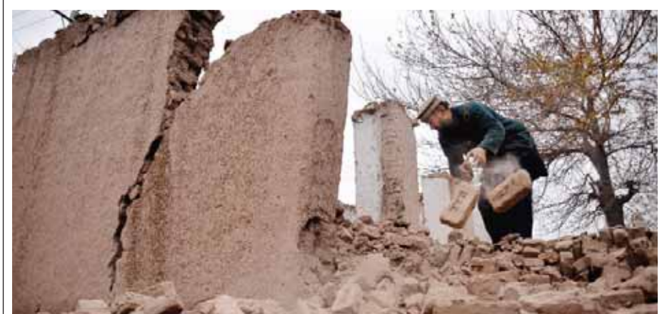
SURKHOAD, Afghanistan: An Afghan villager removes bricks after his home was damaged from an earthquake in this district of Jalalabad east of Kabul yesterday. — AP
