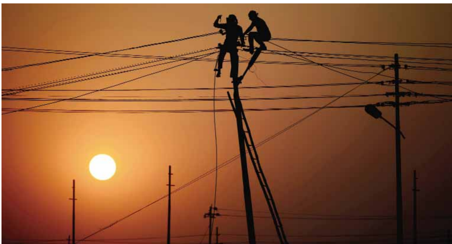
ALLAHABAD: Indian workers adjust electricity cables set up temporarily on the banks of the river Ganga in preparation for the annual Hindu religious fair of Magh Mela yesterday. — AFP
