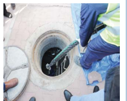
Workers install fiber optic lines as part of Phase two of distributing fiber optic-operated internet in Kuwait.
