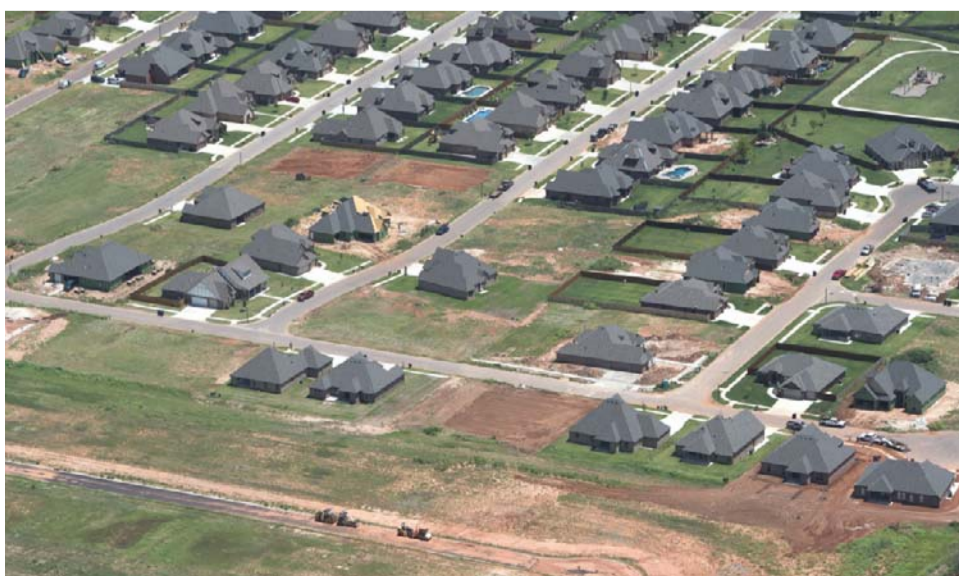
OKLAHOMA CITY: A new home development is seen under construction from the air near Oklahoma City, Oklahoma. New construction of US homes rebounded in November from an October slump and building permits surged as the housing market continues solid growth, official data showed. — AFP
