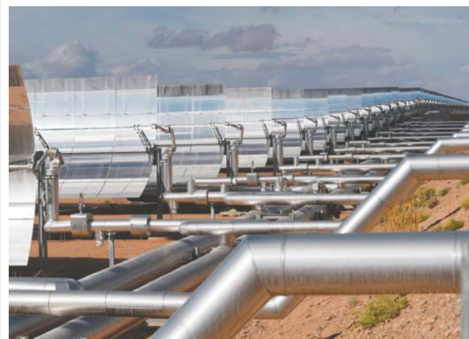
OUARZAZATE, Morocco: A picture taken on Oct 17, 2015 shows a view of the Noor 1 Concentrated Solar Power (CSP) plant, some 20 km outside this central Moroccan town. — AFP
