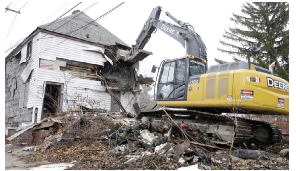
DETROIT: In this photo, an abandoned home is demolished on Detroit's eastside. The city was insolvent in July 2013 when then-state appointed emergency manager Keyvn Orr filed for Detroit's historic bankruptcy. — AP
