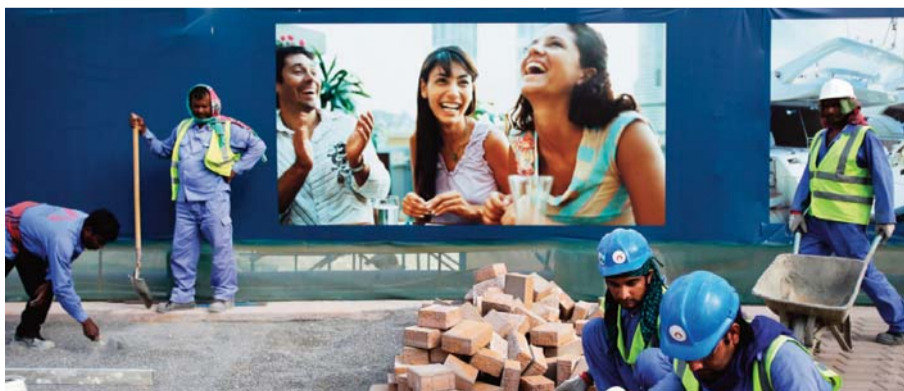
Laborers install paving stones in front of an advertisement for luxury real estate, in the Marina district of Dubai.
