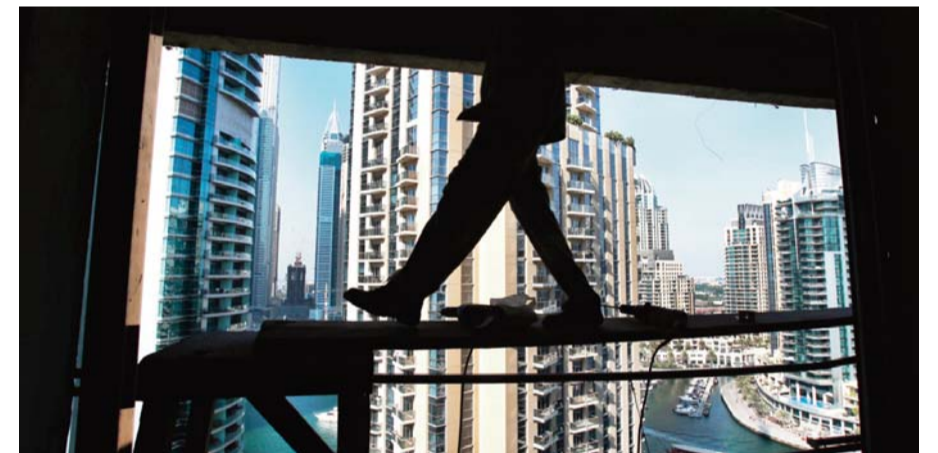
A worker walks on wooden scaffolding while fixing a window frame at a construction site in the Marina neighborhood of Dubai.
