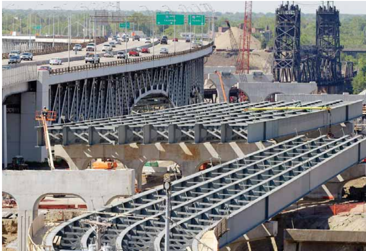
The steel skeleton for the eastern end of the new Innerbelt Bridge in Cleveland sits next to the existing span. The House on Thursday voted overwhelmingly in favor of final passage of a 5-year, $305 billion bill that boosts highway and transit spending and provides states with assurance that federal help will be available for major projects. Senate action is expected to follow shortly. —AP
