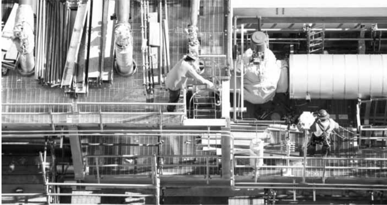
DEKALB: Employees work next to the gas lines of the Mississippi Power Co. carbon capture power plant in DeKalb, Miss. The construction costs for the plant have grown to about $6.4 billion and it has been repeatedly delayed, but Southern Company, owners of Mississippi Power stand by the plant as a model for burning coal while emitting less carbon dioxide and hope to market its key technology. —AP
