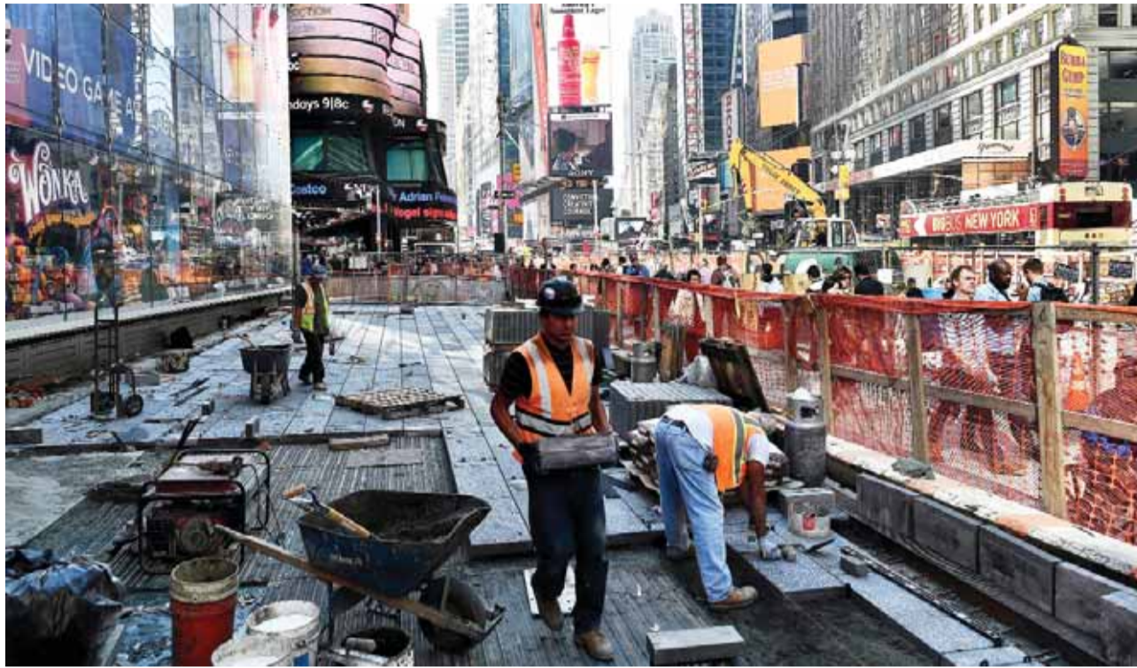
NEW YORK: Laborers work on a footpath and road way construction site in Times Square in New York. The US economy pumped out 211,000 new jobs in November, the Labor Department said yesterday. — AFP
