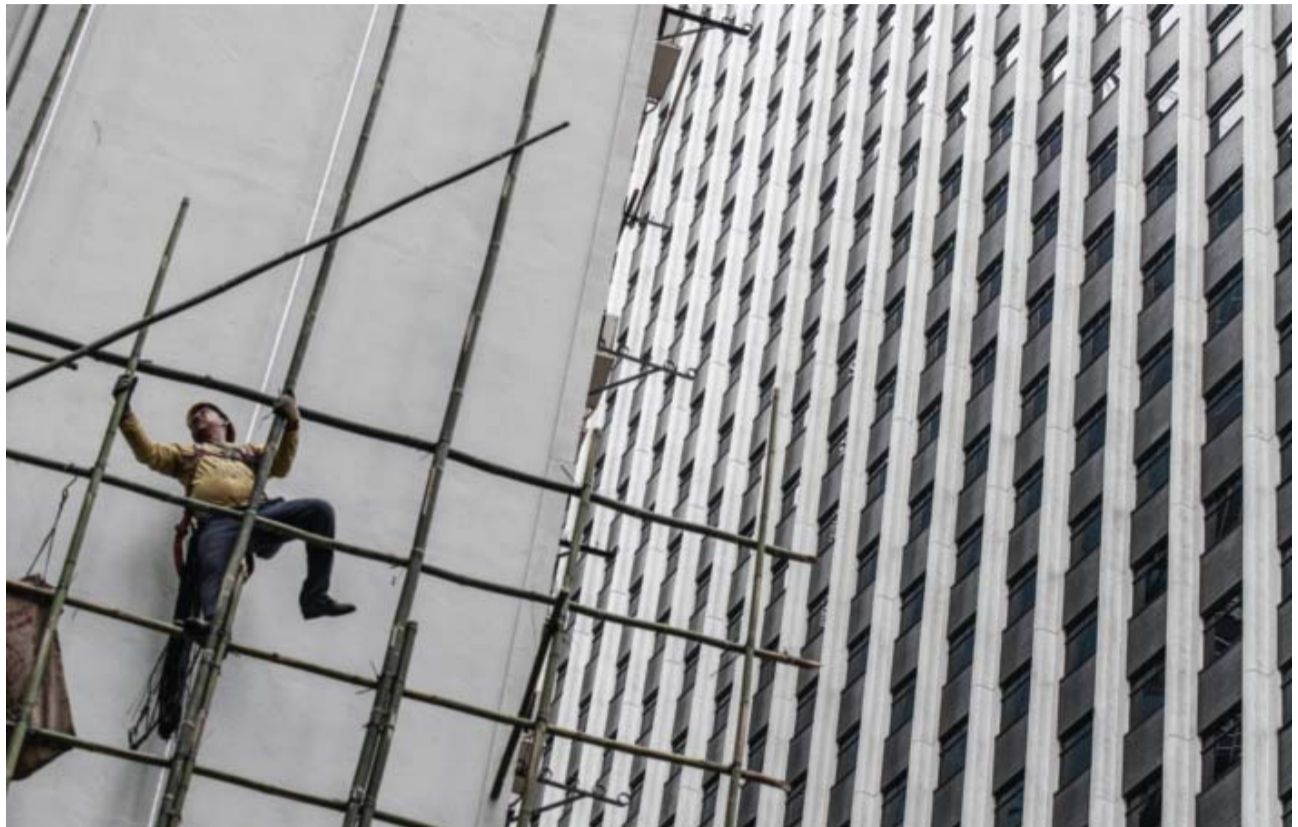
HONG KONG: A worker balances on a bamboo scaffolding in Hong Kong yesterday. Hong Kong's bamboo scaffolders have risen above predictions that their trade would disappear, remaining a common sight high above the streets of the city, scaling the sides of towering, ultra-modern steel and glass buildings on traditional bamboo poles linked through ancient design concepts. — AFP
